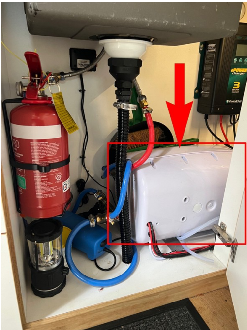
Figure 12 / Hot Water Heater
