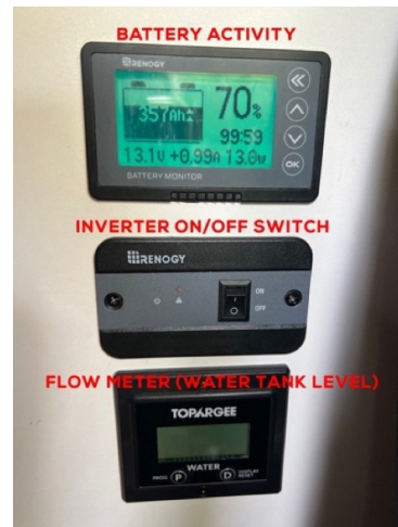
Figure 16 / Inverter Switch (middle)
